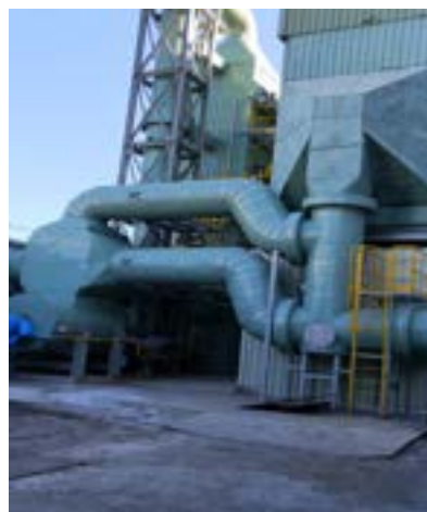
TS-7 SCR denitrification equipment
