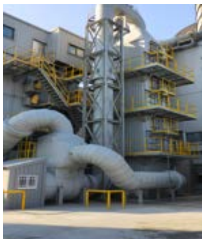
TS-3 SCR denitrification equipment
